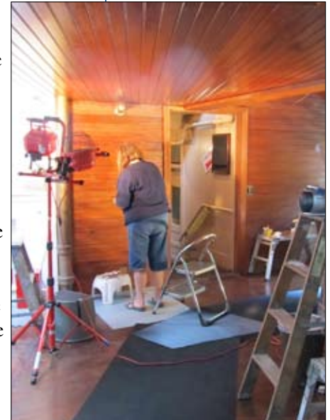
Top: Brigid Sullivan, Chief Conservator, NPS Northeast Museum Services Center restoring the original finish of the cypress washboard paneling in the office entrance.
